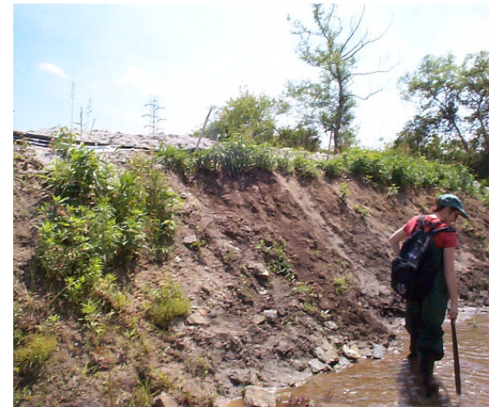
Unstable bank, Dunn Creek, Henderson County
